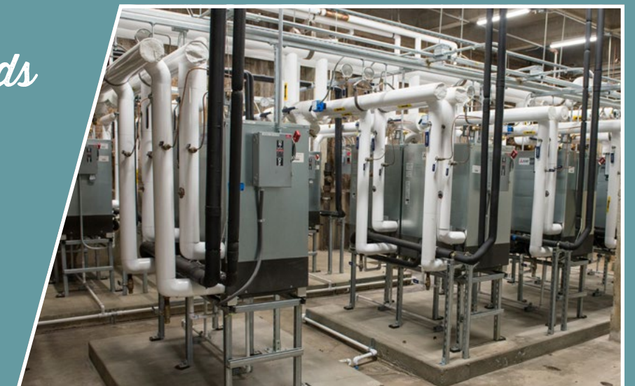
Heat pump exchange units in the Stewart Library.
